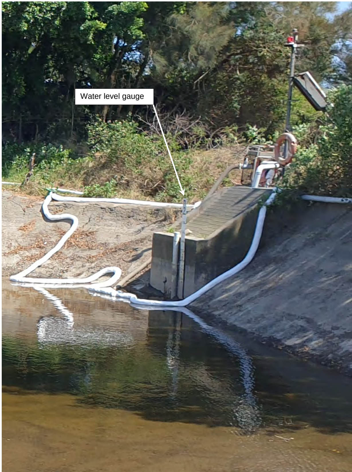
Photo 26 Water level gauge in Final Sedimentation Basin at NW corner of Facility
