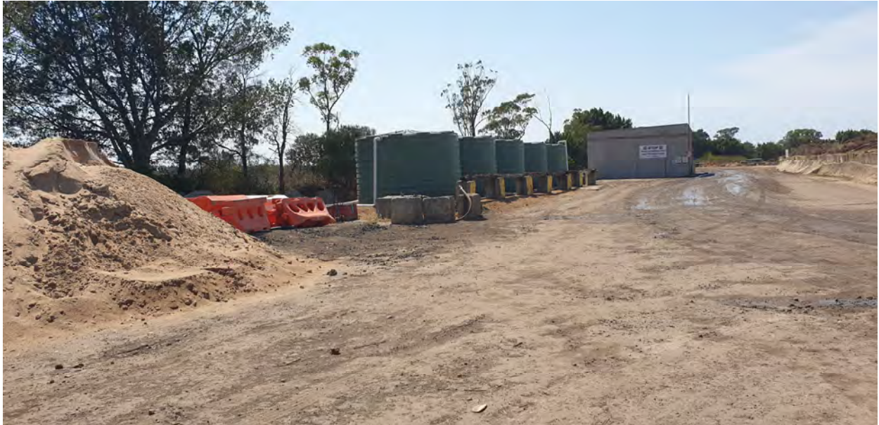
Photo 27 Water holding tanks used for dust suppression in northern end of Facility
