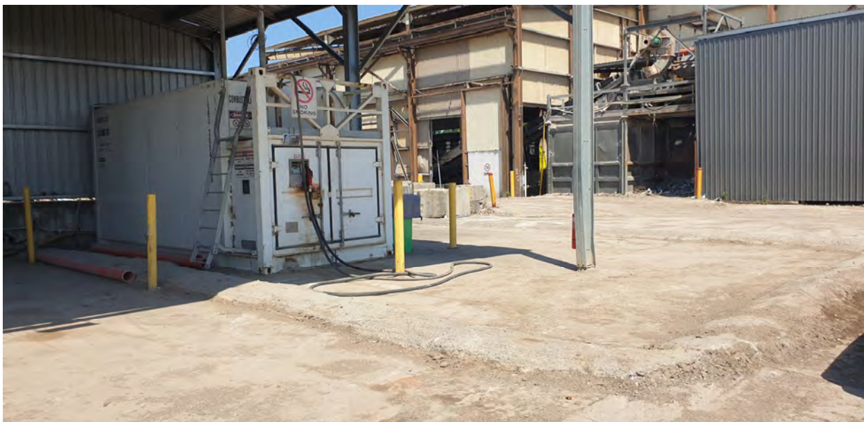
Photo 15 Self-contained 28,750 L diesel AST refuelling facility in bunded area
