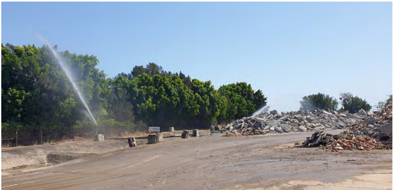
Photo 21 Sprinkler system in operation along western site road
