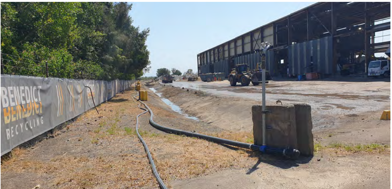
Photo 20 Sprinkler located along western site road
