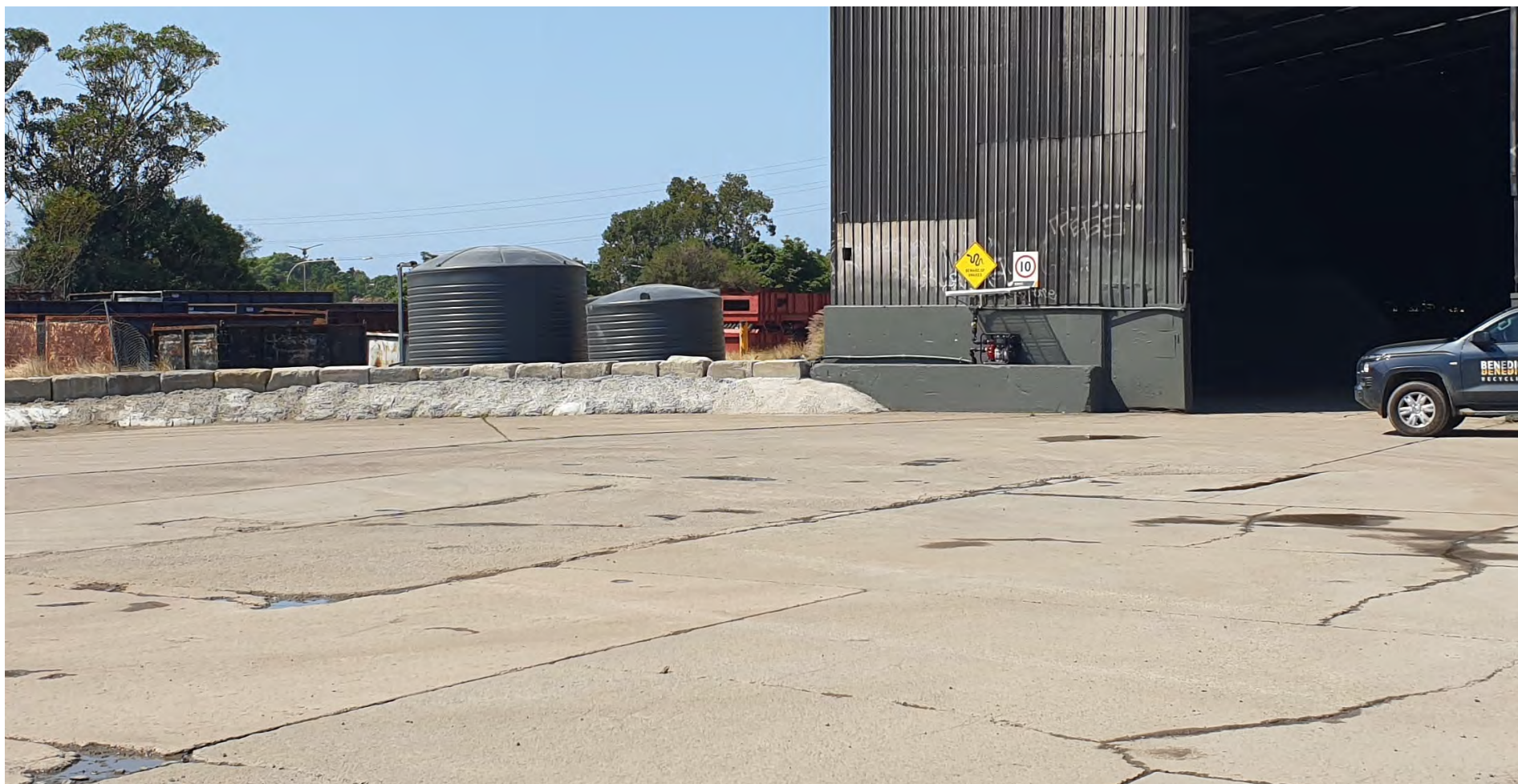
Photo 36 ASS treatment area – surface water storage tanks
