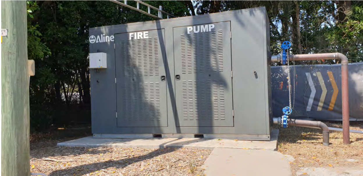
Photo 13 Fire pump at southern end of Facility
