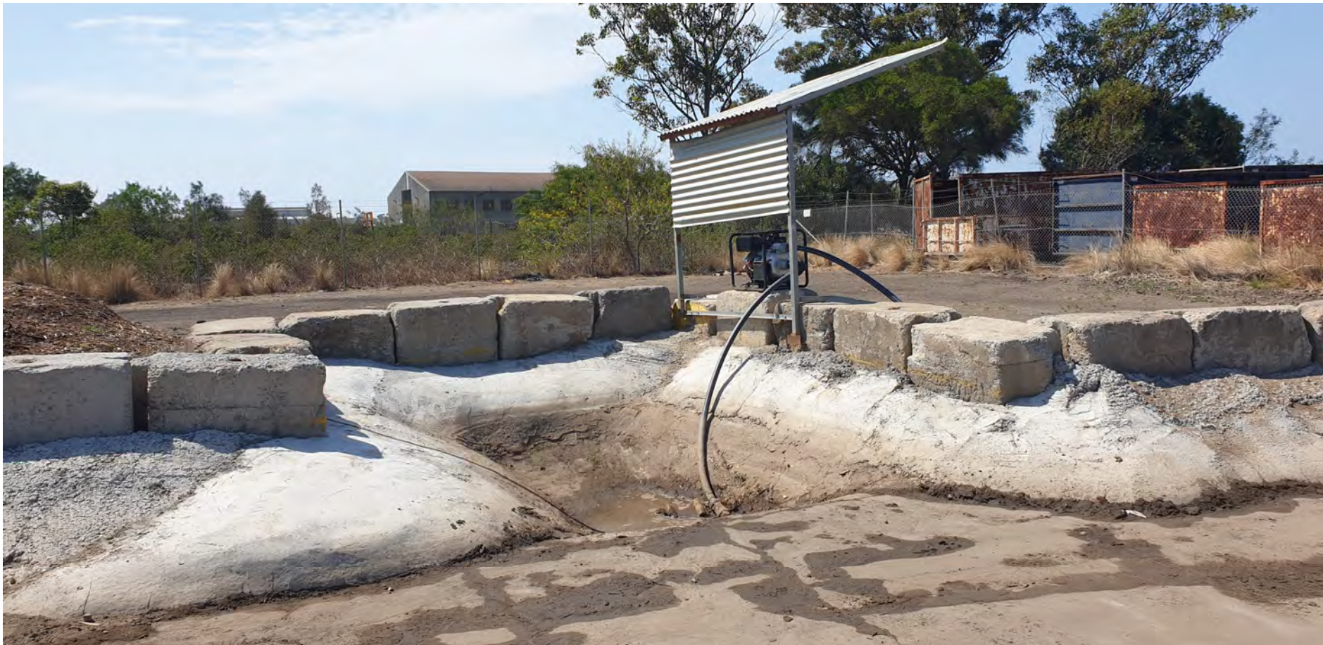
Photo 35 ASS treatment area – surface water drainage pit and pump-out system to storage tanks
