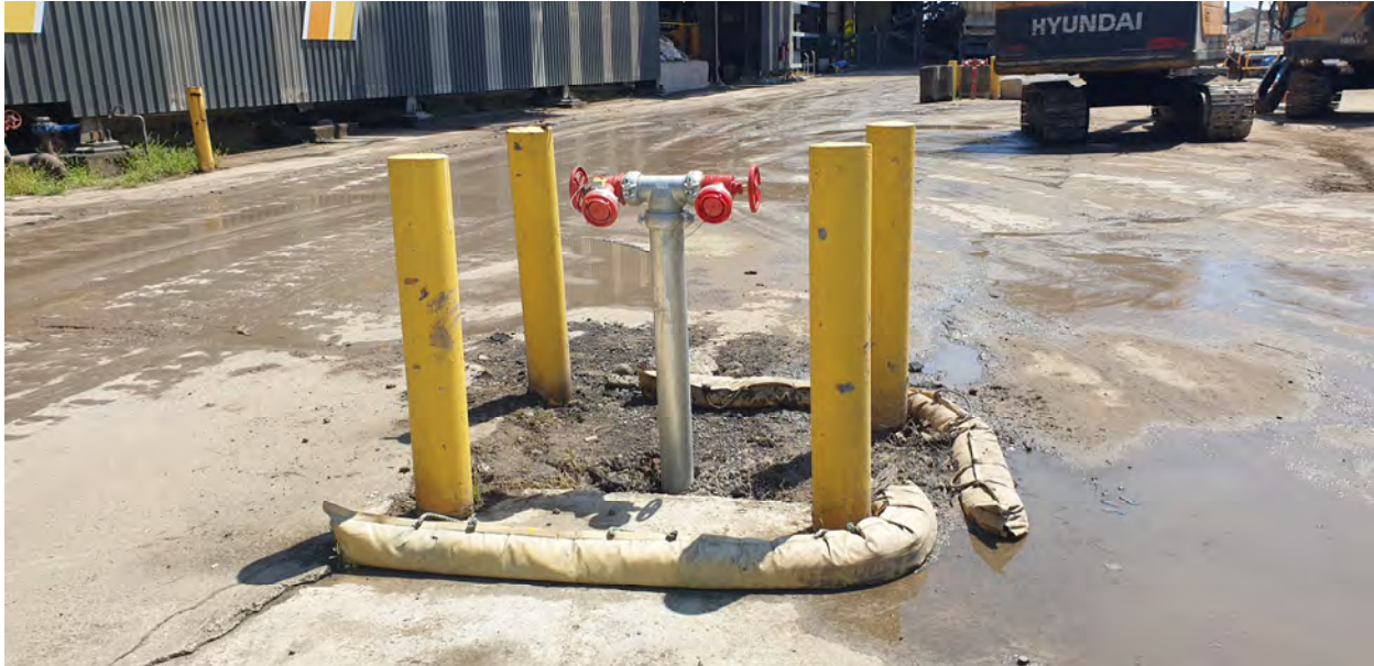
Photo 11 Fire main in central area
