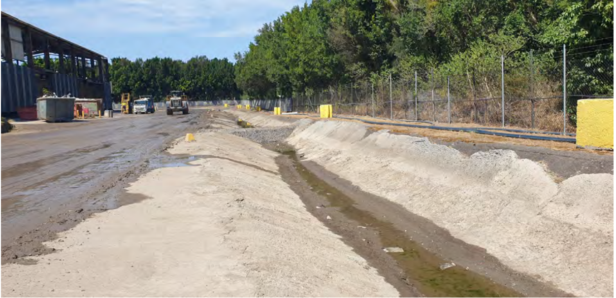
Photo 19 Concrete lined perimeter drain along western side of Facility
