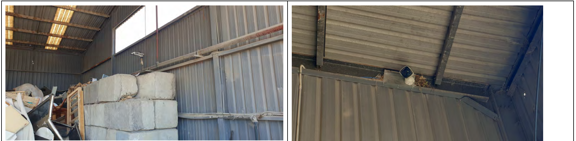
Photo 44 Sprinkler system in Domestic Waste shed
